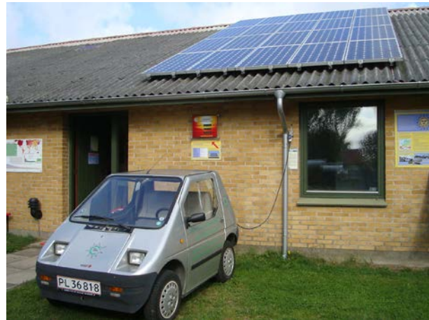
Electric car KEWET is being charged by solar energy at the Folkecenter.
